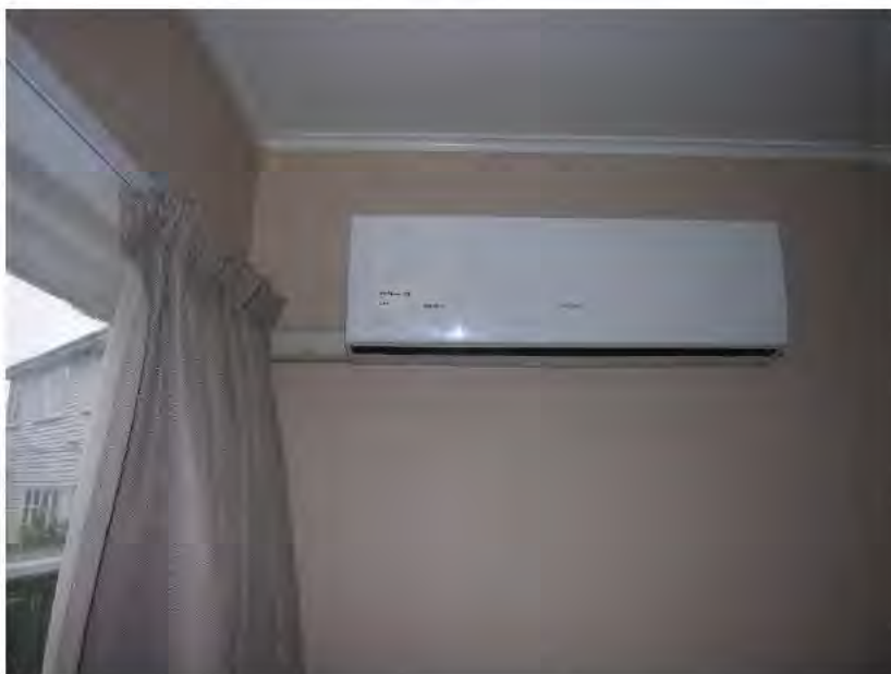
Photograph 6: Sampling site on the heat pump in the lounge.
