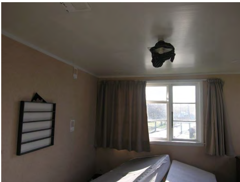
Photograph 7: Sampling sites on the ceiling in bedroom 1.
